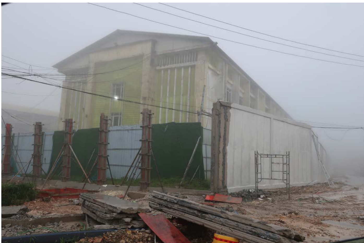
A perimeter wall being constructed around the KA01 compound in mid-2025. This compound was previously abandoned or shuttered in 2023 after police interventions but was confirmed to be active again as of early 2025. © Amnesty International, 2025
